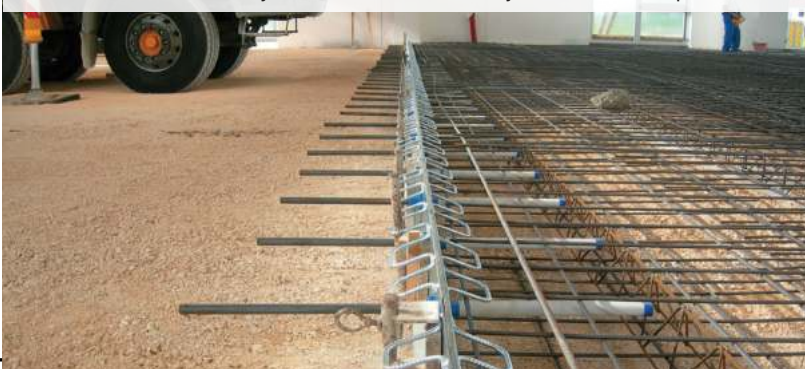
Detail of Ideal Joint System® installed and ready for the concrete placement.
