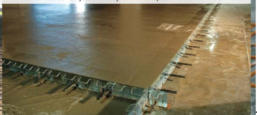
Detail of Ideal Joint System® ready for the next placement of concrete.
